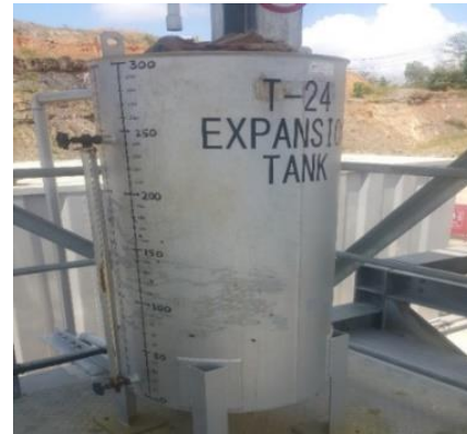
Gambar 5. Expansion Tank 300 L
