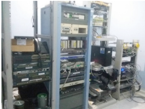
Gambar 3. Ruang Server SNC BPN
